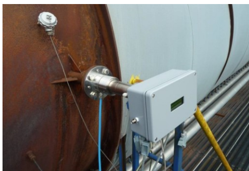
Figure 3. QCL emitter installed at duct.
